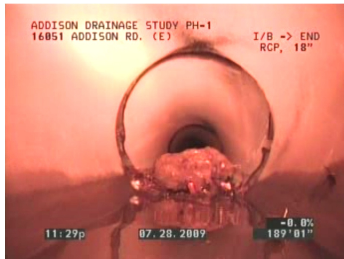
Photo IV-1: CCTV Image of Problem Area in the Keller Springs Branch Basin
