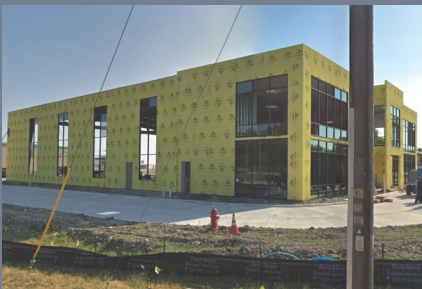
Westgrove Air Plaza II Hangar 4700 Westgrove Drive Two-Story Airplane Hangar with Offices
